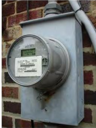
Figura 13. Medidor residencial . https://en.wikipedia.org/wiki/Automatic_meter_reading .
