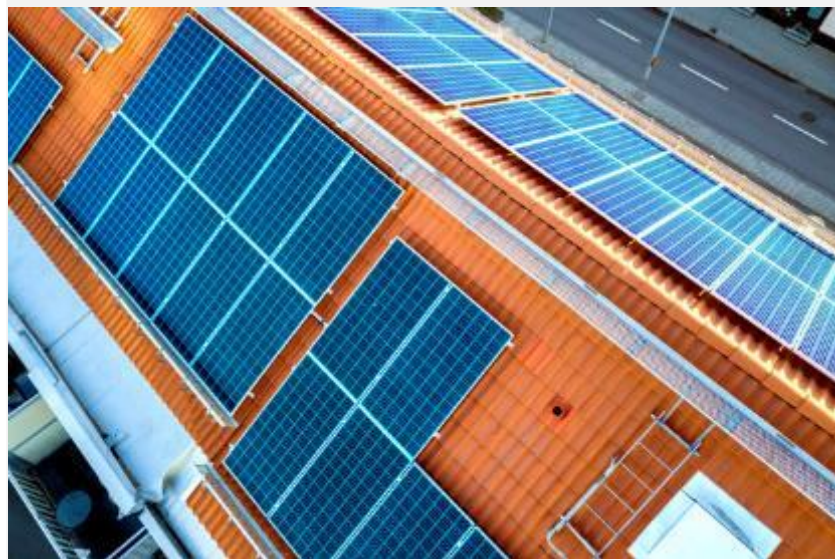
Figura 9 - Modulo Fotovoltaico - Fuente: https://www.freepik.com/premium-photo/top-view-blue-solar-panels-high-apartment-building-roof_5258620.htm
